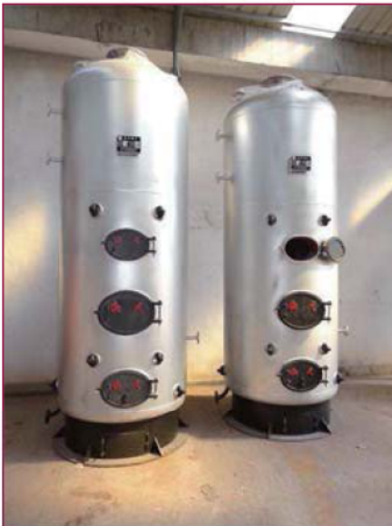
Small boiler circulation
